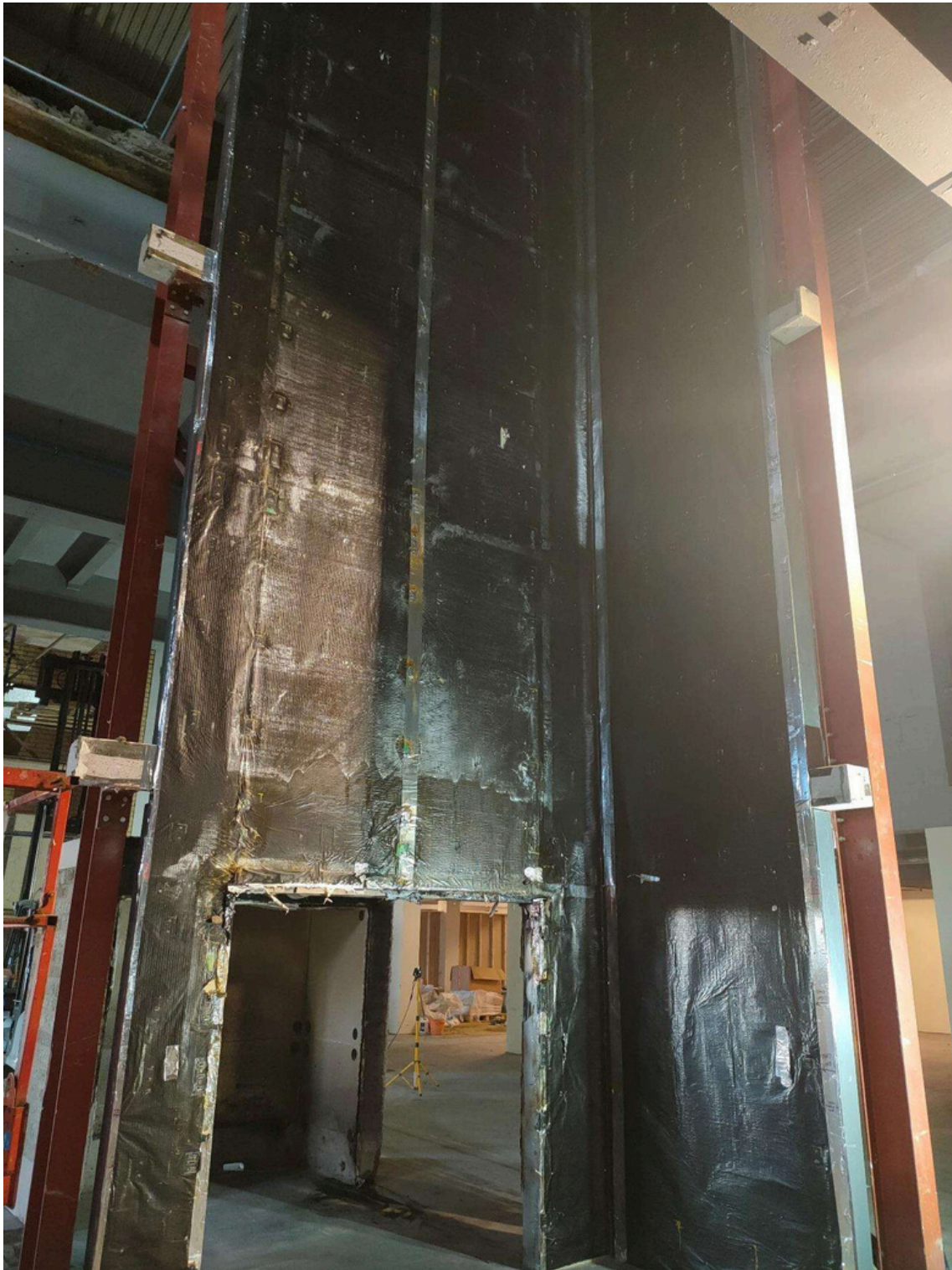
Figure 33. Damage investigation – Air/Vapour membrane after the test.
