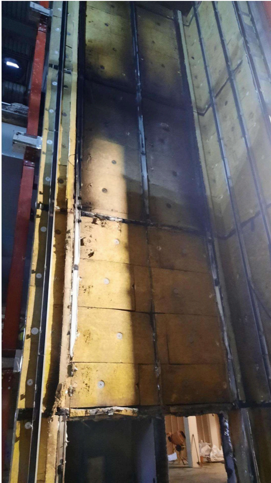
Figure 32. Damage investigation – Insulation and fire cavity barrier after the test.
